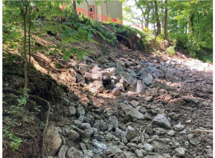
Project site post-construction, showing the installation of large riprap to eliminate the erosion and keep the stream channel from moving closer to the home
